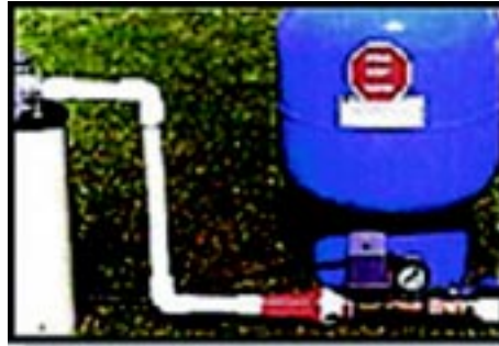
Left: Fourteen gallon tank with a CSV-1... 2 HP submersible runs 2 households and a drip system.
